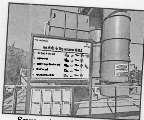
Sewage treatment plant (STP)
