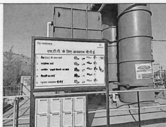
Sewage treatment plant (STP)
