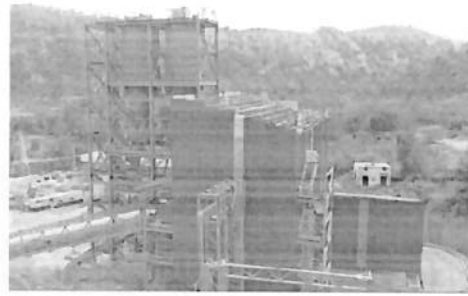
Paste Fill Plant
