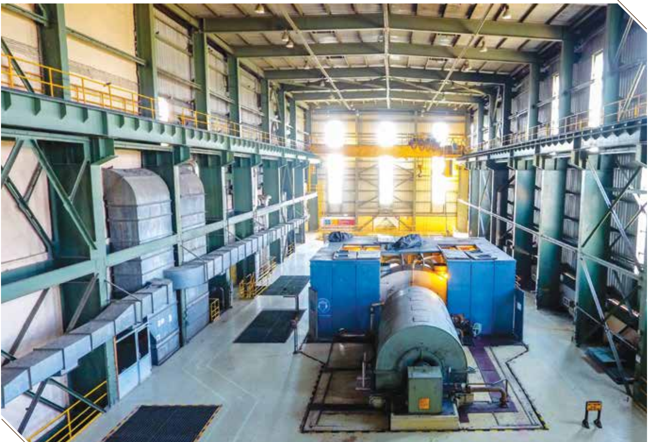
Inside view of turbine area at captive thermal power plant
