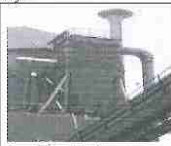
Bag filter, Cyclone at Coal Crusher
