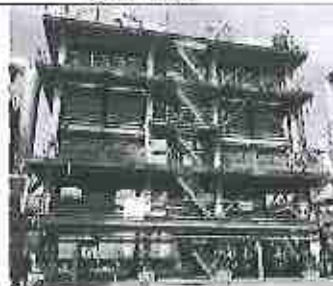
Acid Plant Hot ESP
