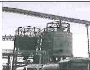
Bag Filter Silo
