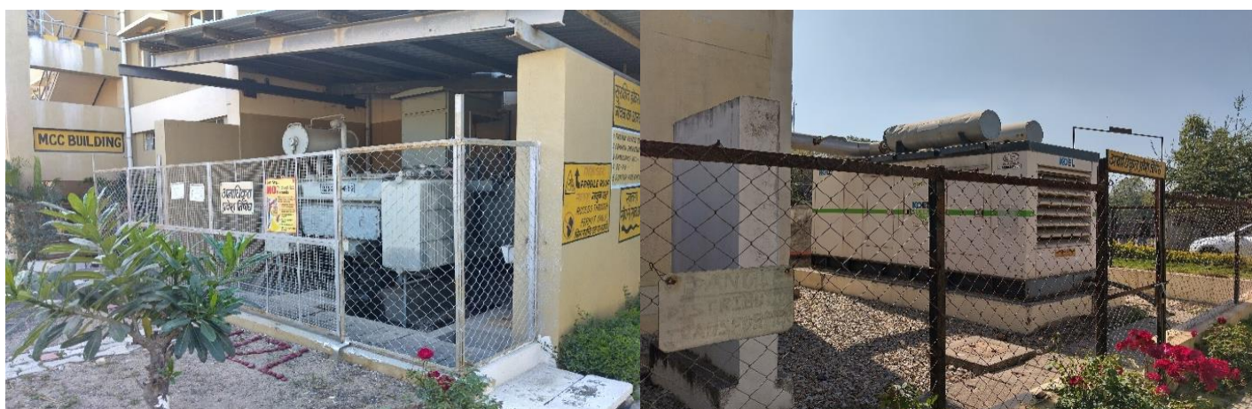
Figure 17 - Power Backup supporting round the clock operations for STPs
