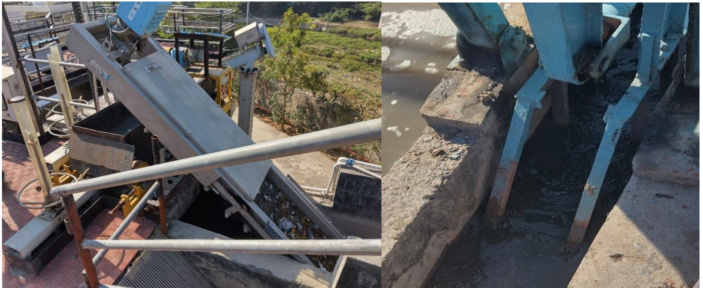
Figure 6 - Stilling Chamber helping in filtration through Grit separator and classifier
