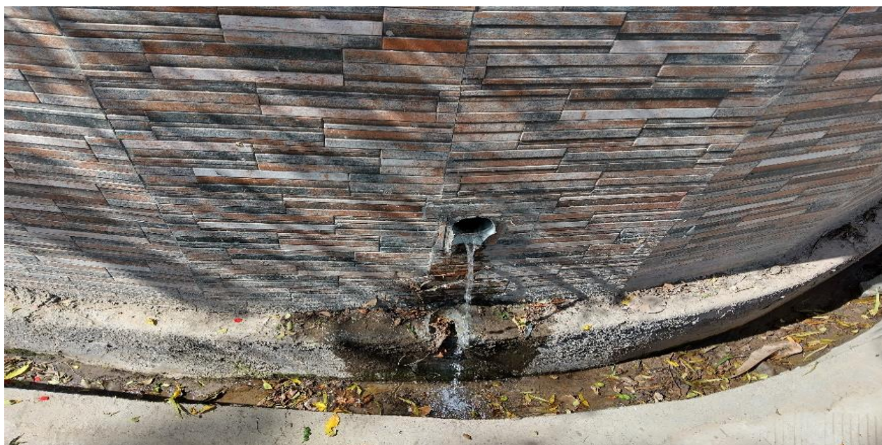
Figure 19 - Waste water leakage in nalas
