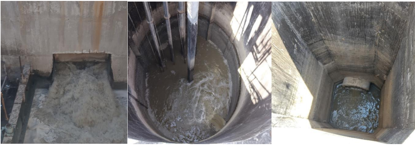
Figure 5 - Waste water entering the STP through inlet
