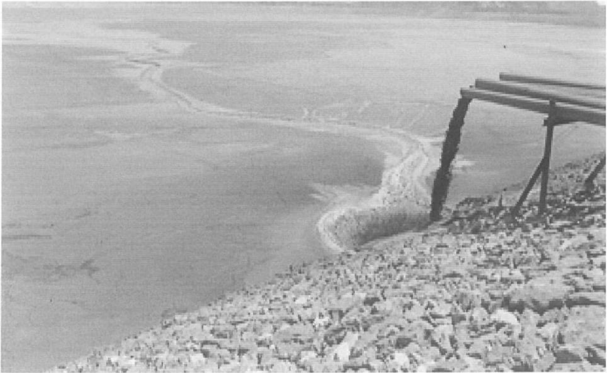
Tailing close pipeline
