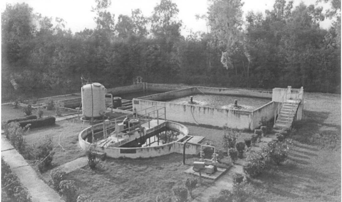
STP (425KLD) in plant premises
