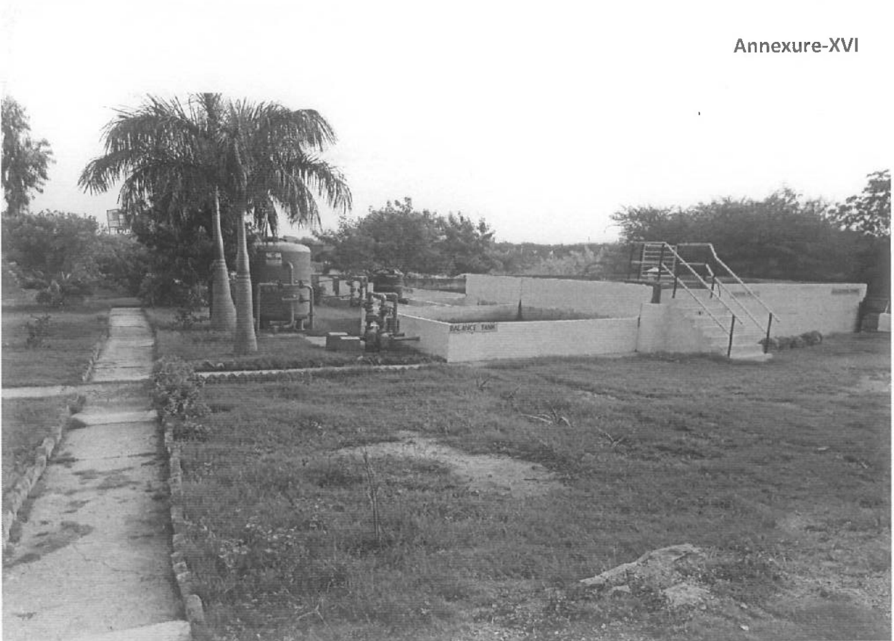
STP (300KLD) in plant premises
