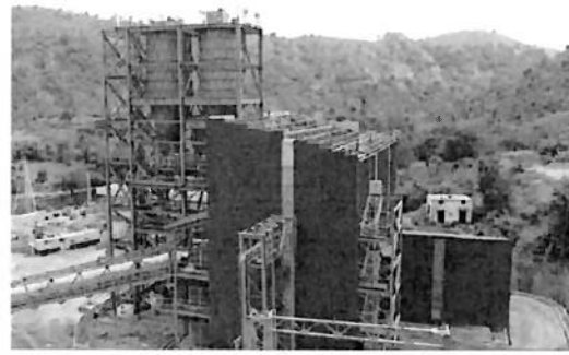
Paste Fill Plant
