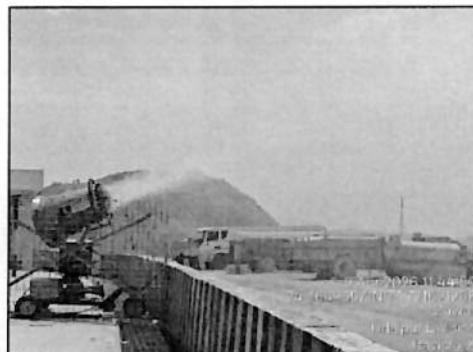
Fogger installation at Adit
