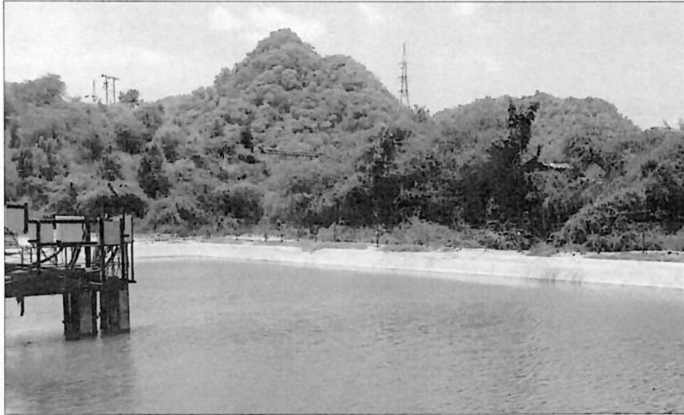
Recycling arrangement (storage cum pumping arrangement)
