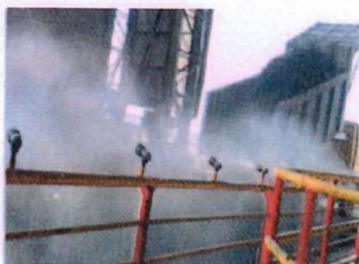
Auto dust suppression system at crusher
