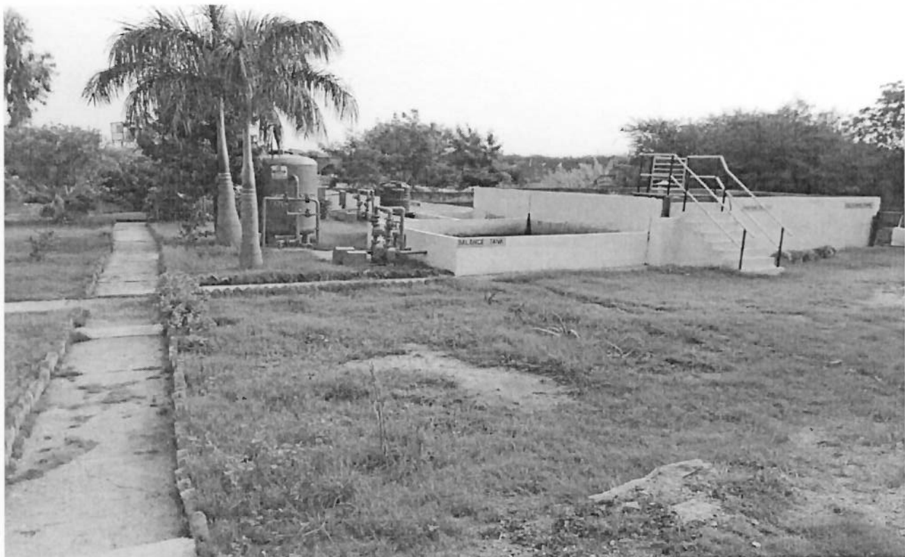
STP (300KLD) in plant premises
