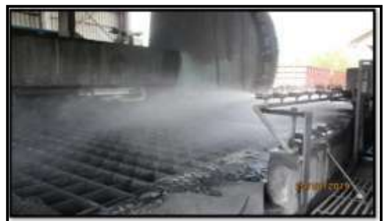
Sprinkler at coal transfer point
