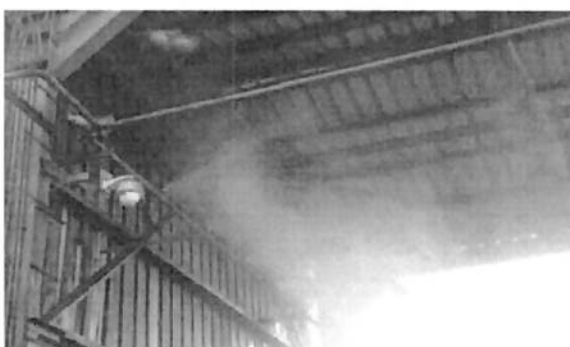
Mist sprinkling system in coal yard
