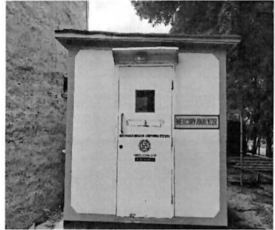
Stack Mercury Monitoring Station
