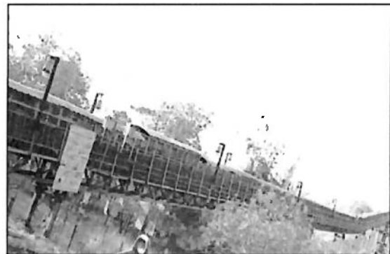
Covered Conveyor Belt
