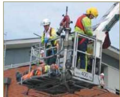
Figure 58: Scaffolder working without a fully-boarded platform
